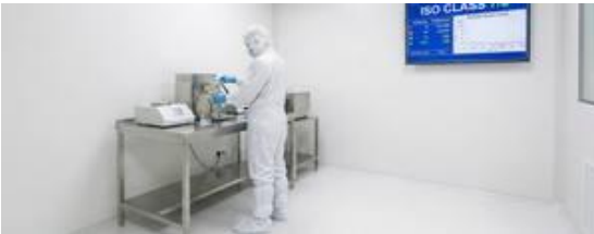
Clean room / GMP Rooms added without altering the frame
